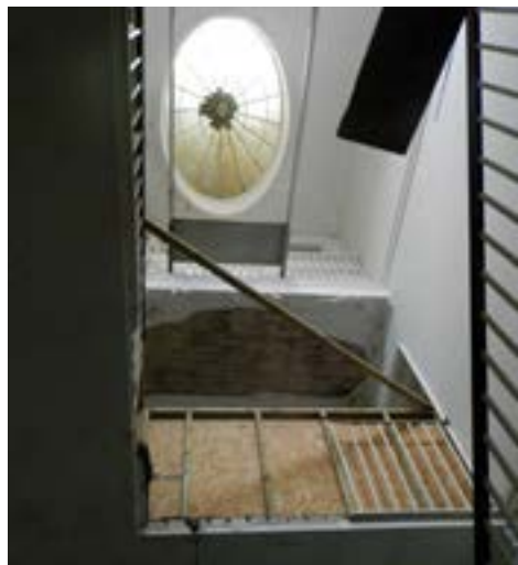
Main stairwell at risk
